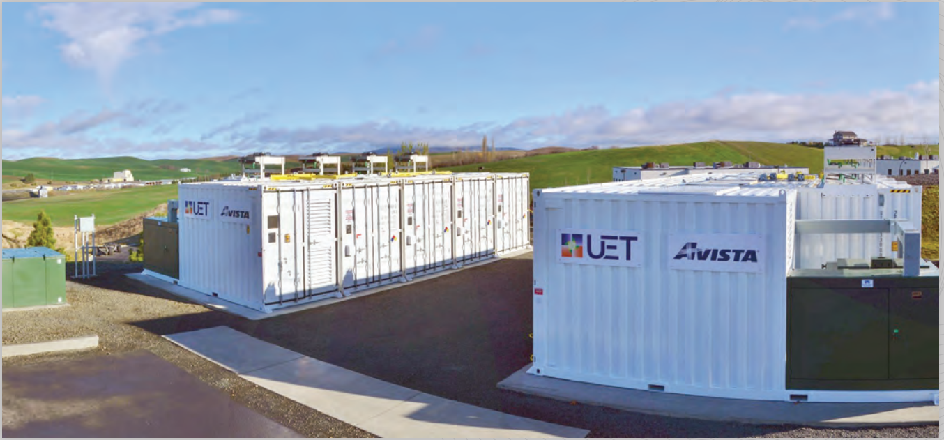
The 1 MW AC /4MWh AC Uni.System installed at Schweitzer Engineering Laboratories in Pullman, Washington
